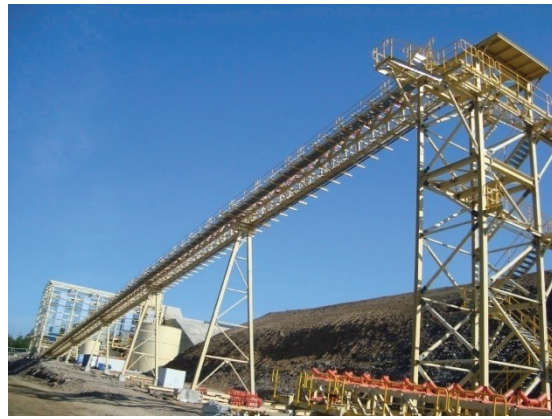
b) Belt conveyer with high-rise trestle
