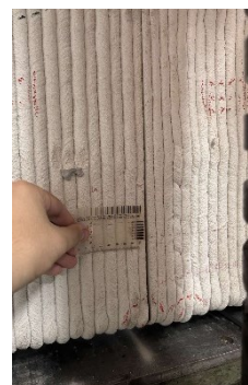
Figure 18. The gap between segments
