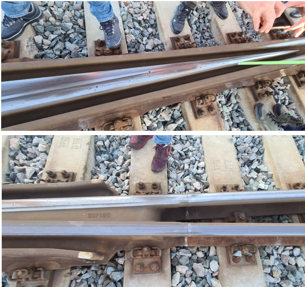
Figure 3. Belgrospi cracks forming on the corrugation peaks in the switch on the Stara Pazova – Novi Sad railway line (Photoby Aleksandar Milutinović in December 2023)
