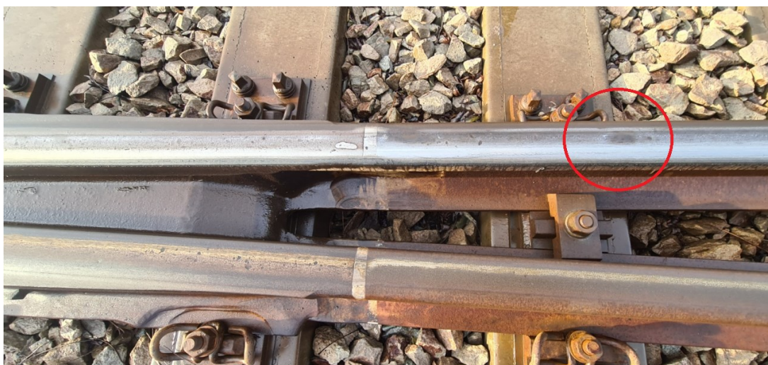
Figure 4. A squat defect developed right next to the concrete sleeper (Photo by Aleksandar Milutinović in Indjija station, December 2023)
