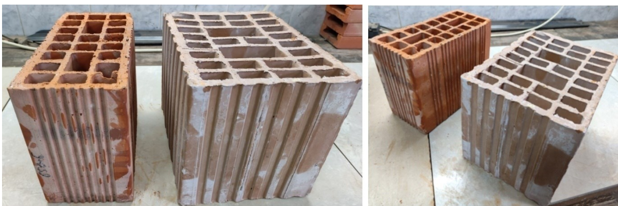
Figure 4. Macroscopic appearance of the samples containing sulfate scum
