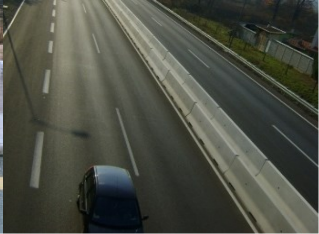
Figure 2. Safety barrier built of SCC-NCA, highway Banja Luka –Gradiška, after 12 years of exploitation
