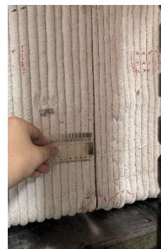
Figure 18. The gap between segments
