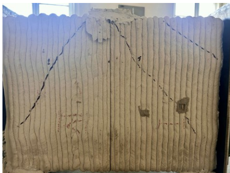
Figure 15. The failure mechanism of the segmental beam in 3-point test – front side
